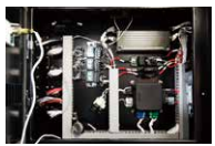
Centralized electric cabinet 集中式电控箱
